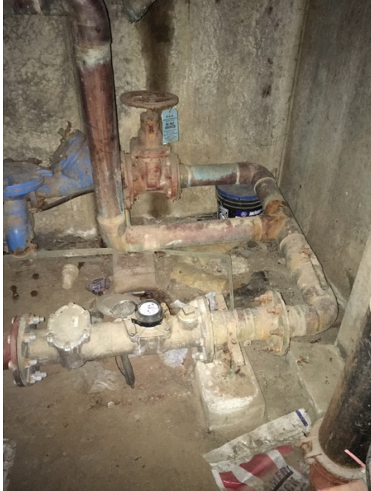
Figure 3 Incoming water service
